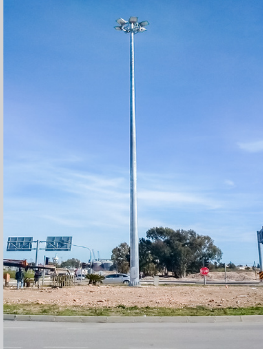
Highmast with Camera
